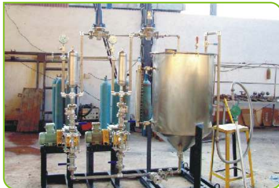
Additive Dosing Skid
